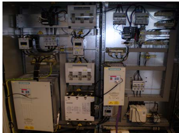
Figure 3: Photograph of Part of the Motor and Generator Power Electronics Circuitry.
